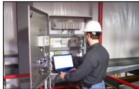
ECT provides full field service support, from checkout to commissioning and remote support for system troubleshooting.
